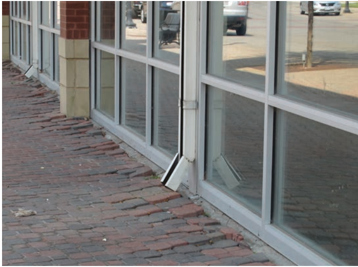
Figure 17. Differential brick settling at the Promenade Theatre. Source: authors.
